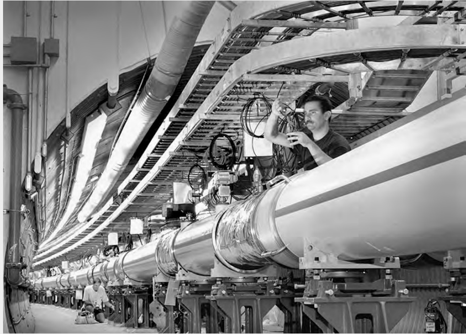
Superconducting magnets at the Relativistic Heavy Ion Collider, Brookhaven National Laboratory.
